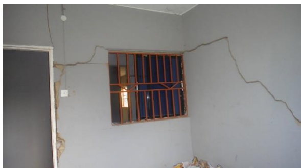
Figure 3: Cracks in one of the rooms
