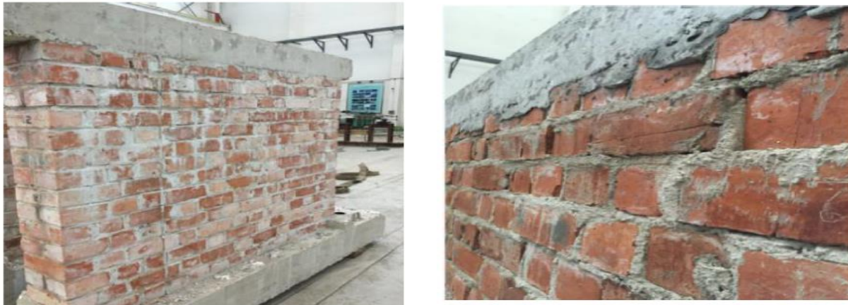
(a) The wall turned white after fire exposure
