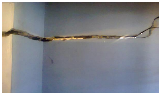
Figure 2: Sign of differential settlement
