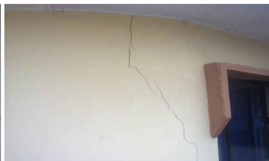
Figure 4: Cracks on the outside wall
