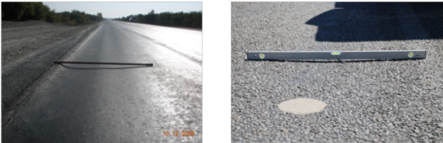
Figure 20. Settlements and consolidations in the chip sealed road pavements
