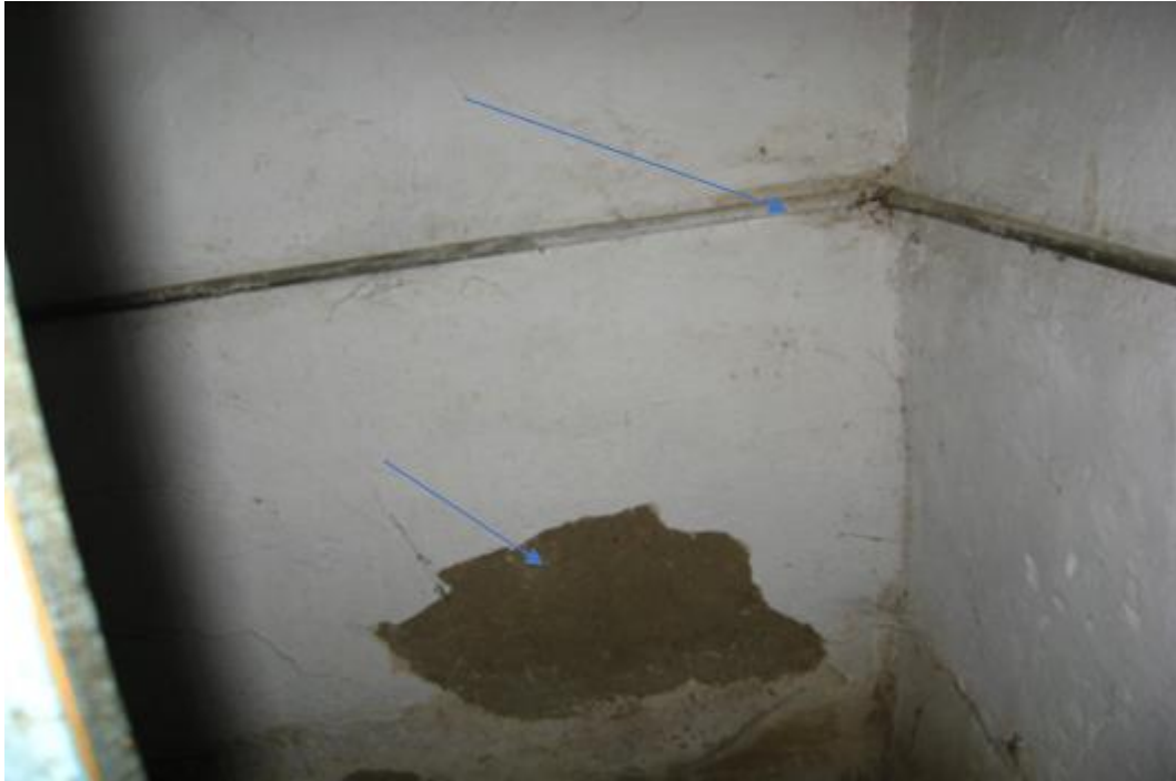
Figure 10. Ayşe Sezgin House of deterioration of the wall surface due to water and moisture.
