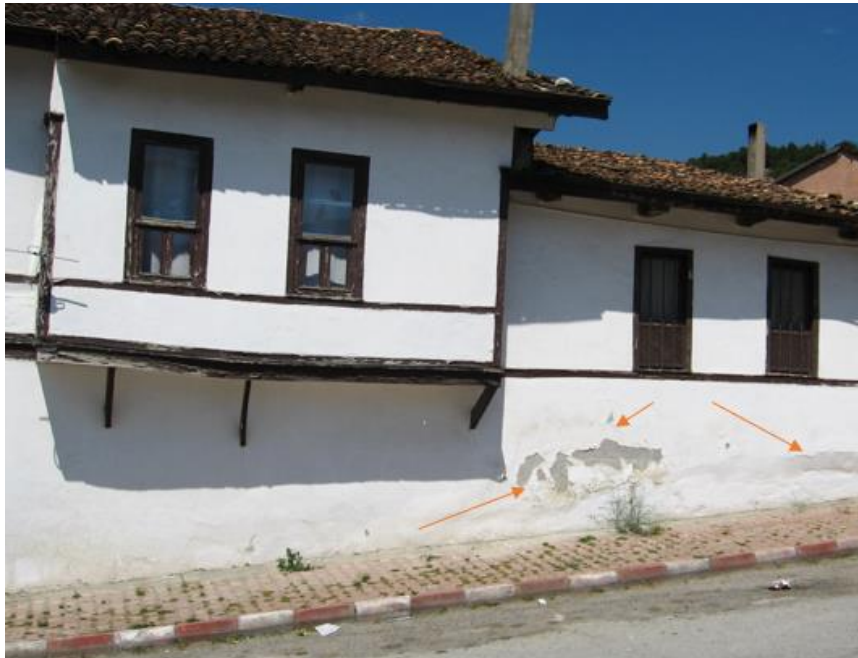
Figure 7. Nevzat Akay House of deteriorations caused by the effect of heat on the exterior of the sturcture.
