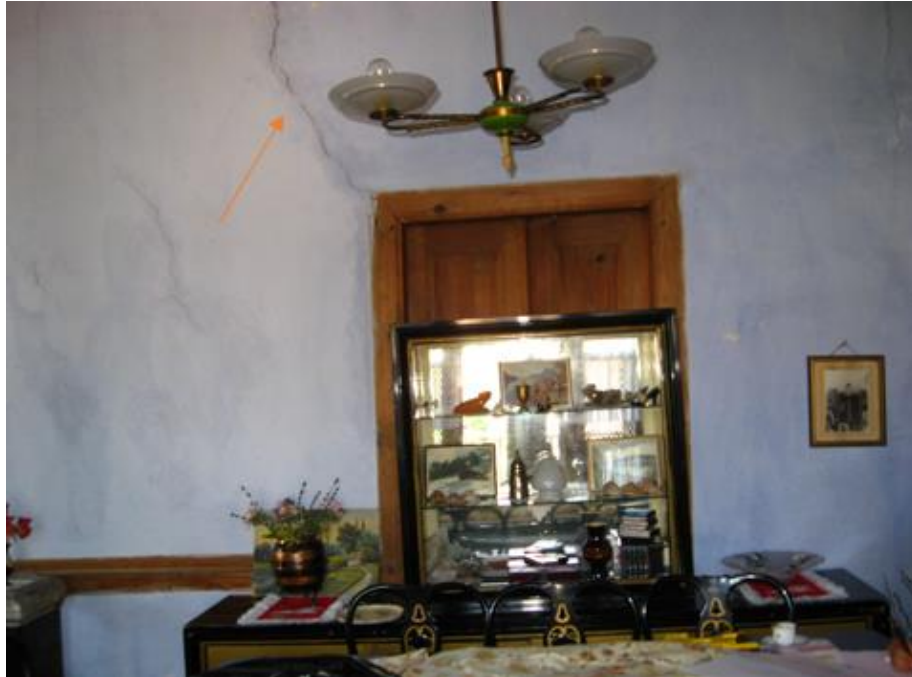
Figure 12. Ayşe Sezgin House of crack caused by mechanical action on the wall surface.
