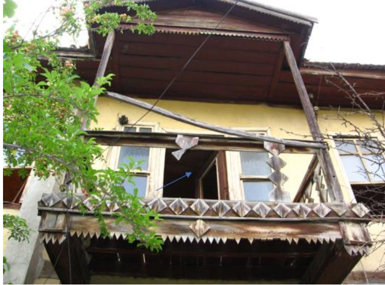
Figure 4. İbrahim Pilavcı House of breaks in balcony railing due to mechanical effect.
