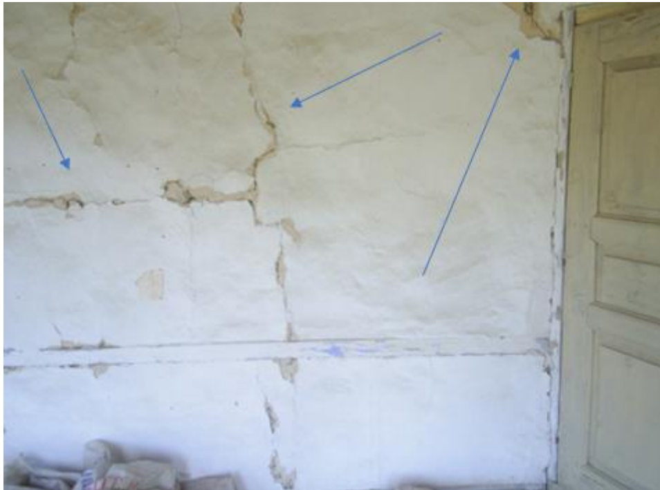
Figure 15. İbrahim Pilavcı House of crack caused by mechanical action on the wall surface.
