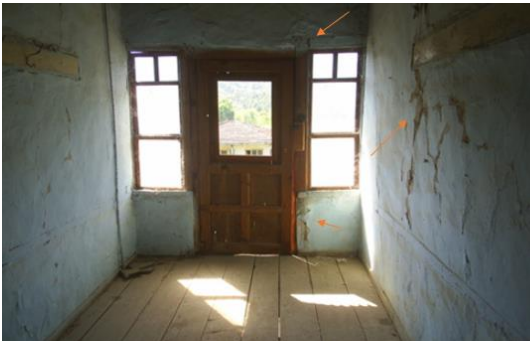
Figure 17. İbrahim Pilavcı House of crack caused by mechanical action on the wall surface.
