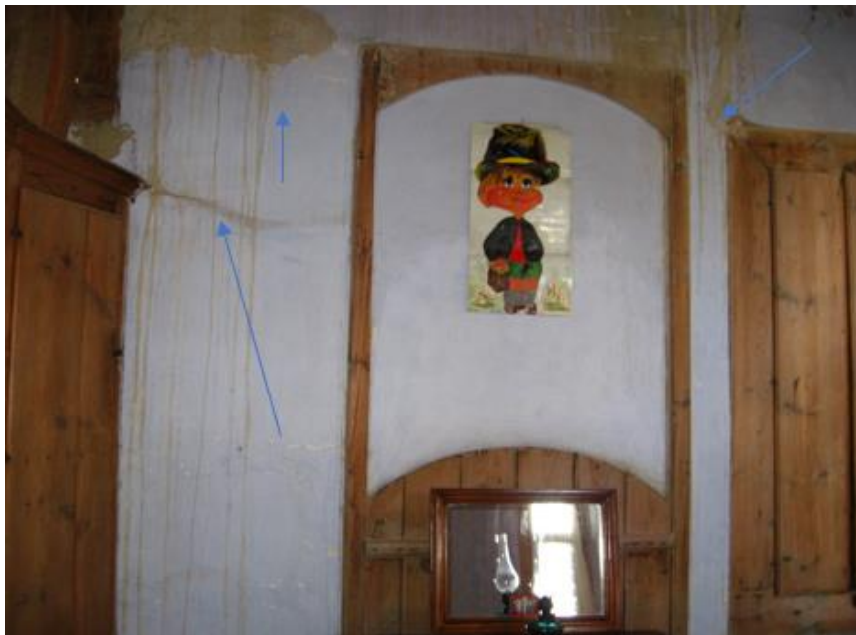
Figure 9. Ayşe Sezgin House of moisture formation on the wall surface due to water and humidity.
