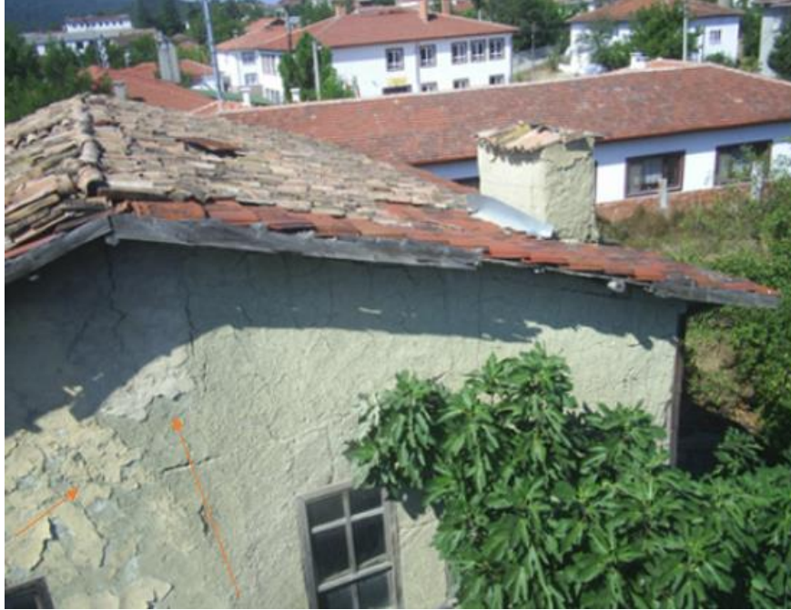
Figure 6. İbrahim Pilavcı House of deteriorations caused by the effect of heat on the exterior of the sturcture.
