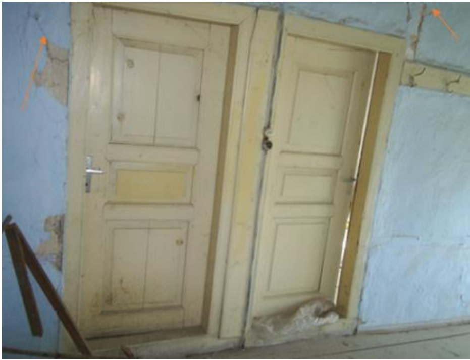
Figure 14. İbrahim Pilavcı House of crack caused by mechanical action on the wall surface.
